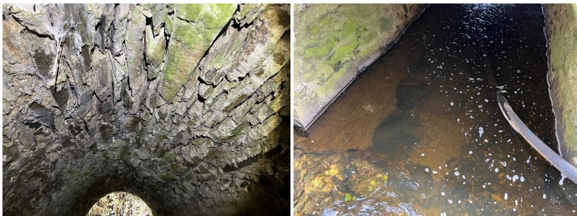
Figure 3-1 – Pointing and masonry loss to the masonry arch barrel (L) and scour damage at the south elevation (R)
